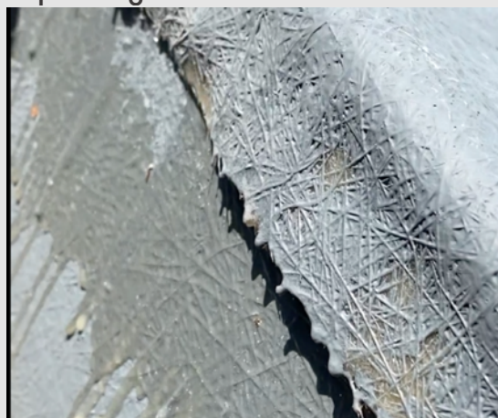
Poor coverage around perimeter
