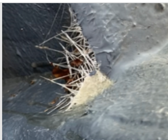
Exposed glass fibres
